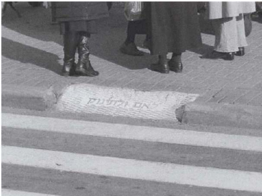
Picture 2. Unsuitable and uncomfortable lowered curb.
